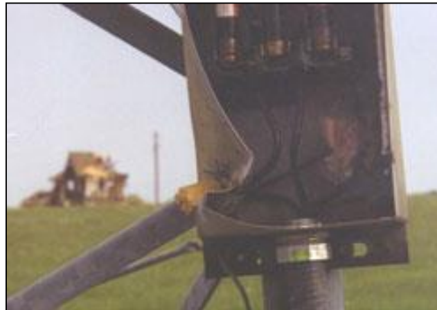
Wood penetrating steel enclosure on turbine tower, May 3 rd , 1999 Moore, OK tornado
